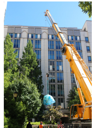
A towering rig lifted the 20-ton Gamma Knife off a flatbed and maneuvered it into position.
