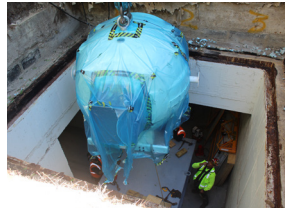
An access hatch was opened to allow the machine to be lowered into the sub-basement, then maneuvered to its destination in the Stitch Radiation Oncology Center.
